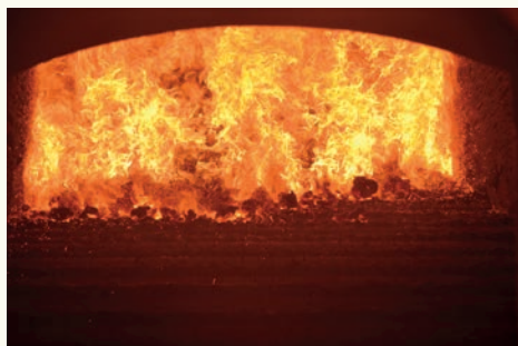
Blick in die Brennkammer
